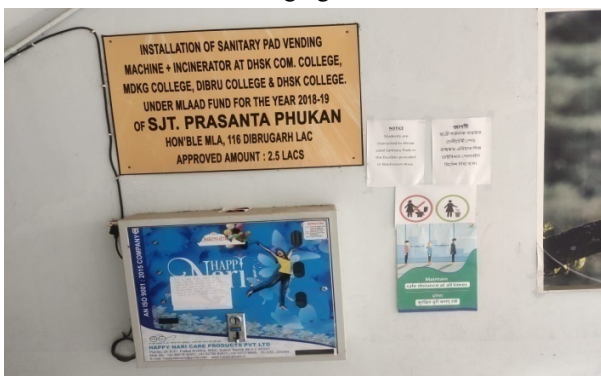
Sanitary pad vending machine and incinerator
