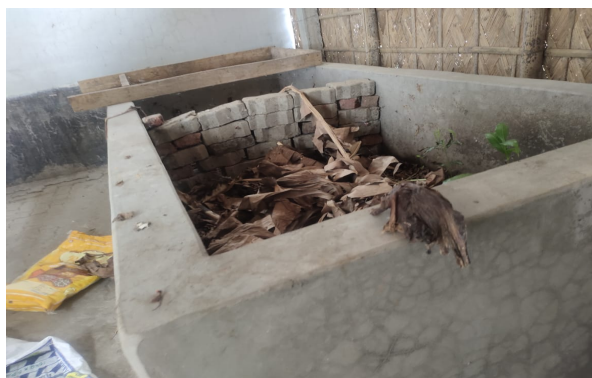
Vermi-composting unit in the college campus
